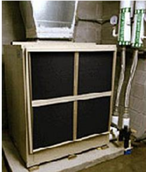
Geothermal heat pump system on the Georgia Institute of Technology Campus Courtesy of U.S. DOE, Craig Miller Productions
