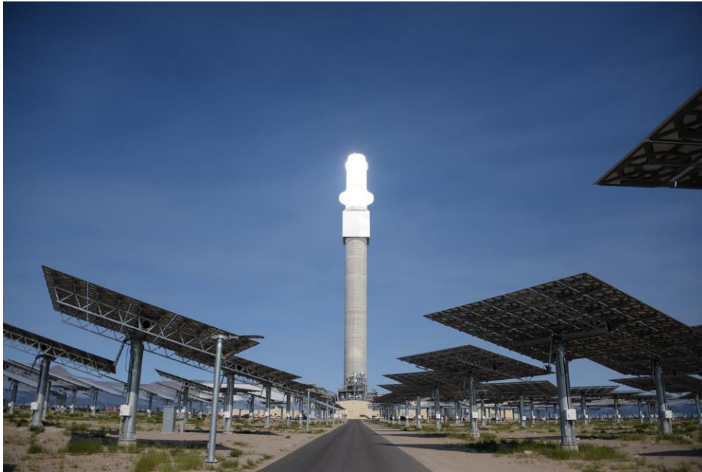
Large tracking mirrors, called heliostats, follow the sun throughout the day, reflecting and concentrating sunlight onto the top of Crescent Dunes' central tower. Credit: SolarReserve
