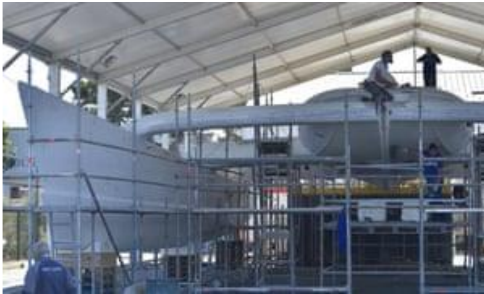
Work on the hull of the Energy Observer in Saint Malo, western France. Photograph: Loic Venance/AFP/Getty Images
