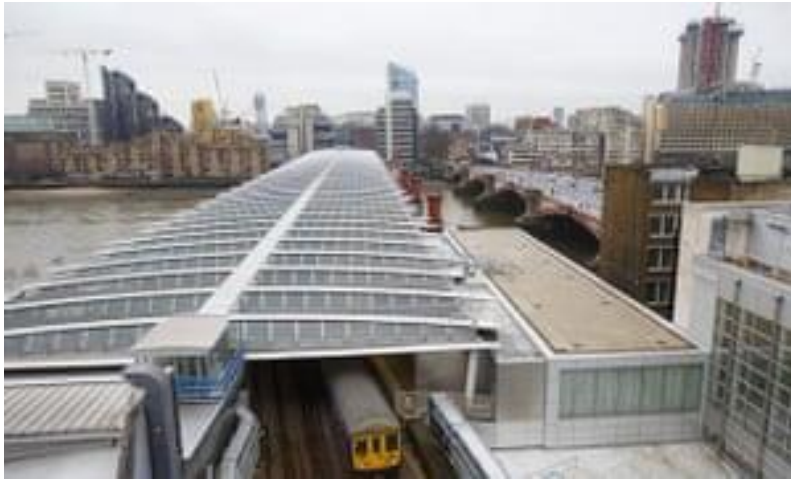
The completed installation of solar panels at Blackfriars station. Photograph: /Network Rail
